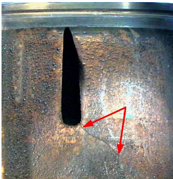
A 2 Crankcase crack in the area of the cylinder liner
